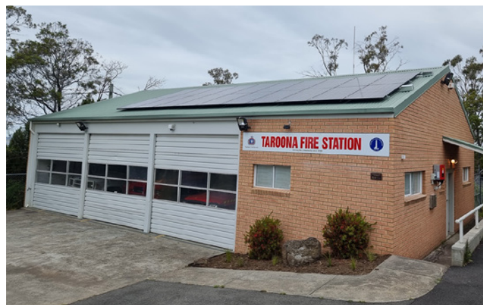
The newly installed 7.4kW rooftop solar power system. The system was gifted to the Taroona Volunteer Fire Brigade by the Taroona Community Association.
