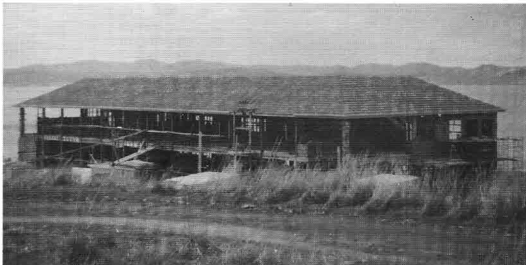
"A" Block just after the completion of the roof, 1957. PHOTO GRACE DIXON.
